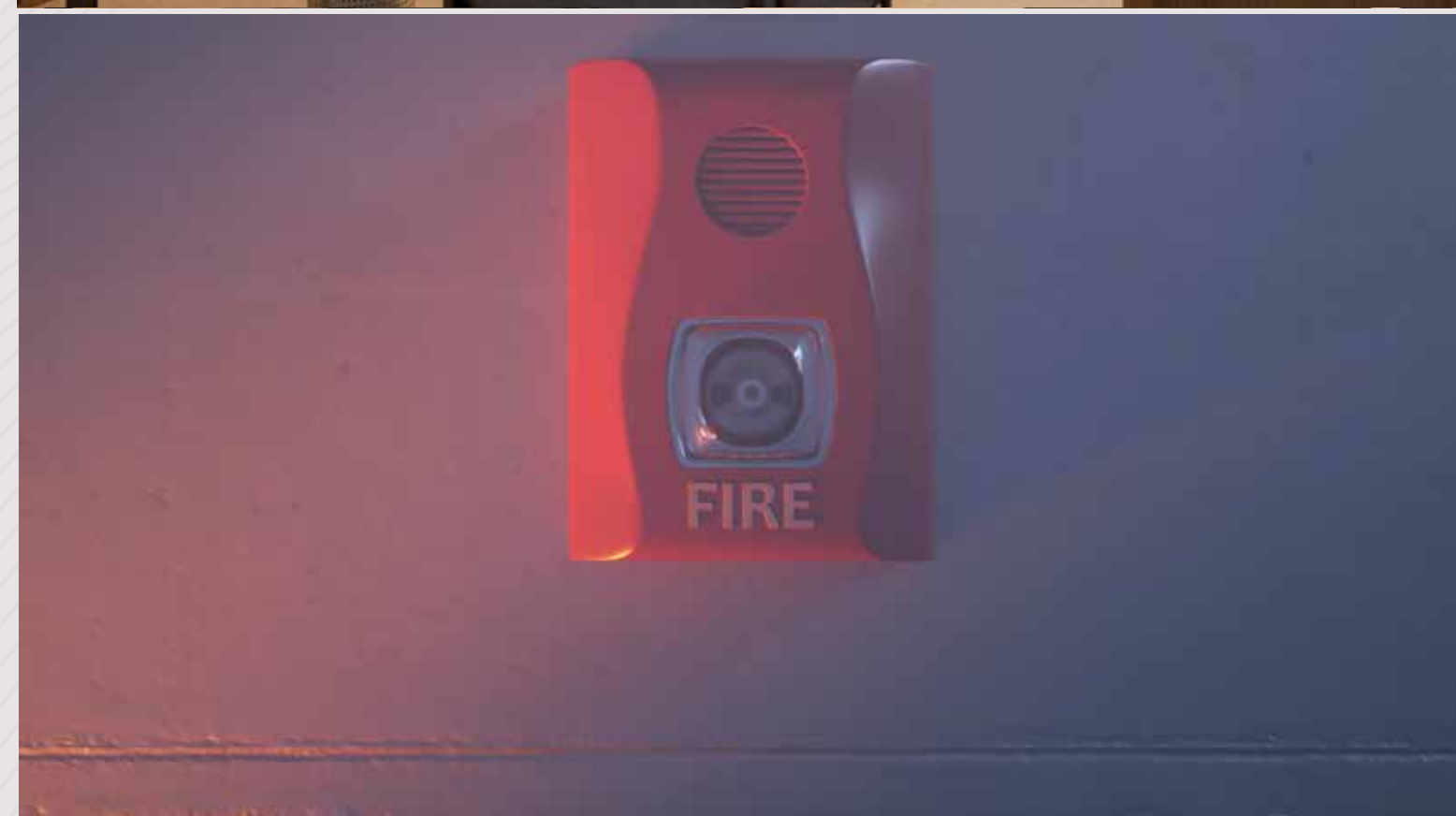
FIRE FIGHTING SYSTEM
